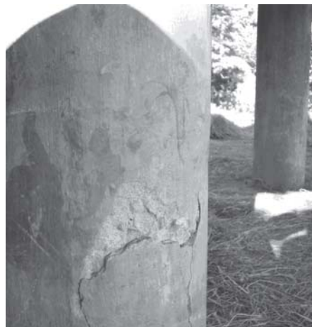
Crack has appeared on the pillar of Cyclone Shelter from earth quake in Moheshkhali; Picture: 13 th November 2005.
