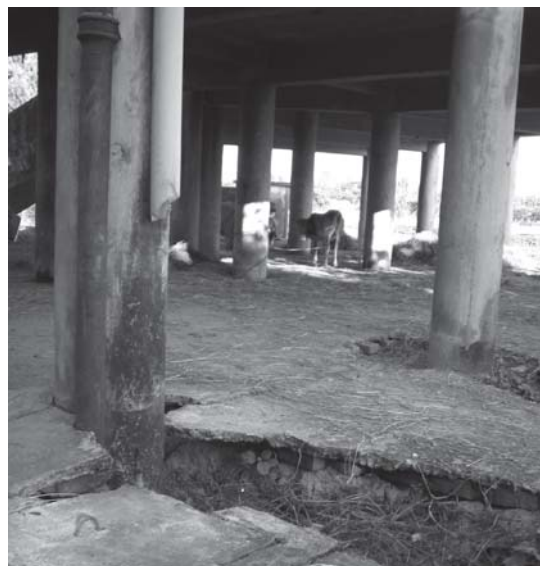
Crack at the basement of Talipare Cyclone Shelter in Moheshkhali; Picture: 12 th November 2005.
