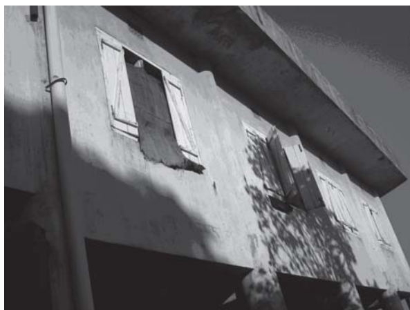
There are no proper windows at the Cyclone Shelter of Moheshkhali; Picture: 12 th November 2005.
